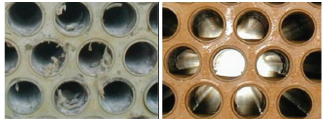
Figure 8. Condition of the brine heater on acid dosing and new HT-antiscalant
