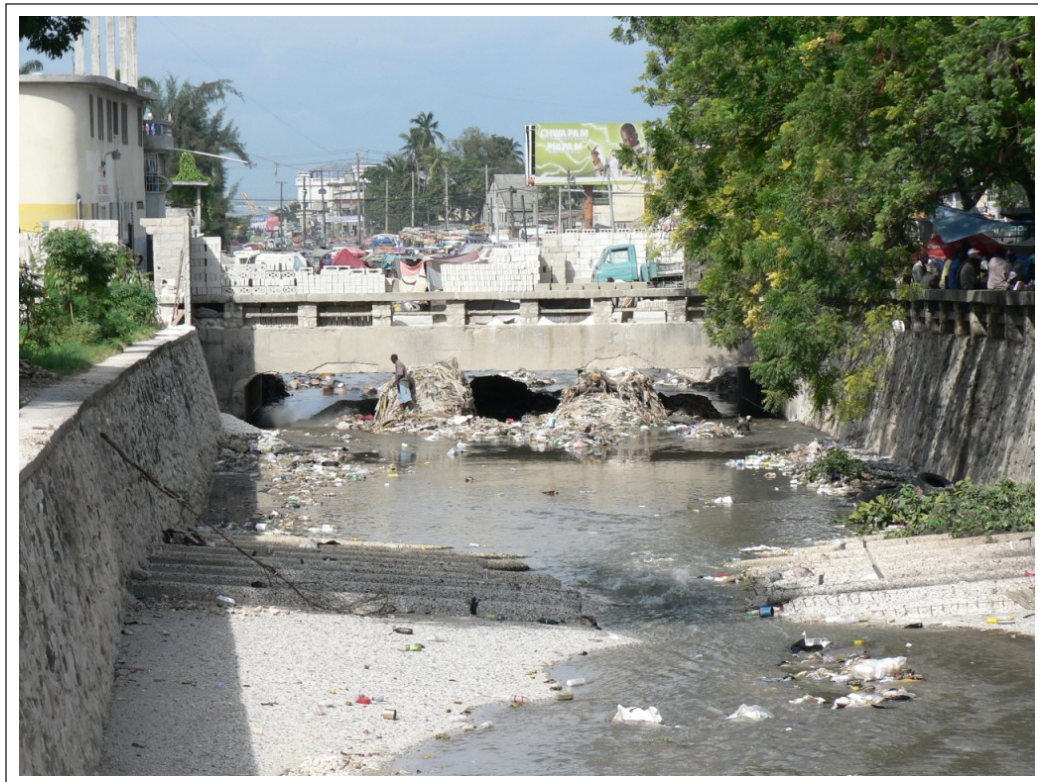
Image 1. Environmental impact that generates in an urban area a channel of discharge of rainwater combined with black waters, Prince Port, Haiti. (Photographer: Alfonso Gutiérrez 2005)
